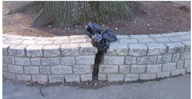
Figure 3. Broken brick barrier and trash found on the path between Frog Pond and baseball fields.
